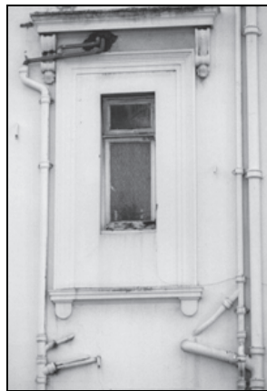
Excessive pipework (and inappropriate window) spoil this building
